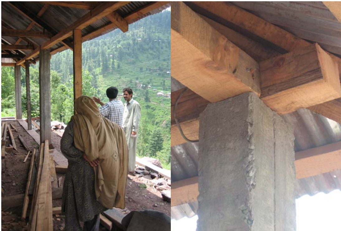
Picture 8. Eastern edge of residential area near the mountains. Sloped terrain. New construction site (after the earthquake).
