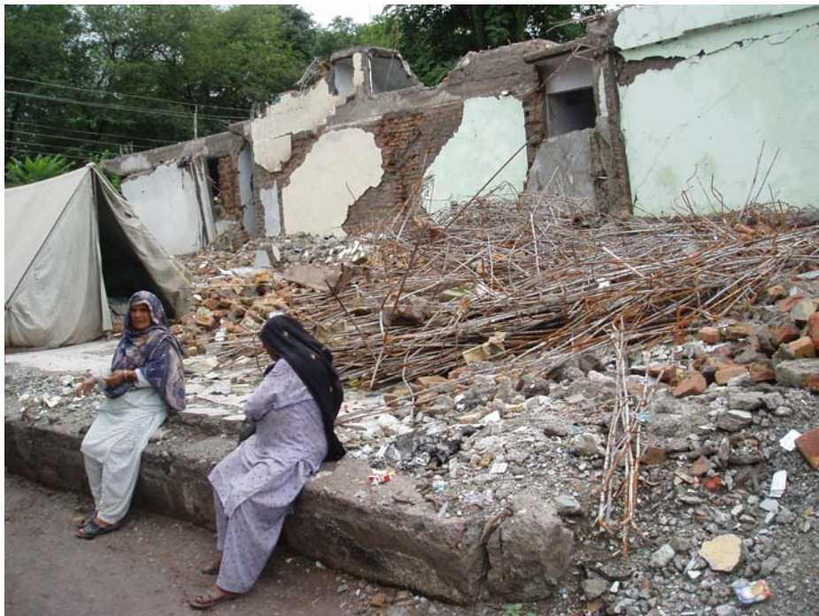
Picture 2. Old part of city near ancient ruins. Standard bricks. 30-70 years old. Original building was 3 stories tall; only parts of back wall remain. The metal rods were not part of the original building that collapsed. Flat terrain.
