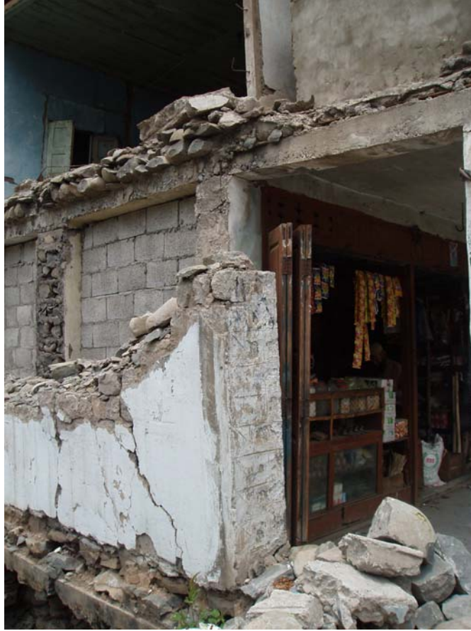
Picture 5. Center of residential area. Collapsed front walls were stacked brick and stone mixed with cement and mortar. Remaining structural walls were all intact. Gently sloping terrain. 10-30 years old.
